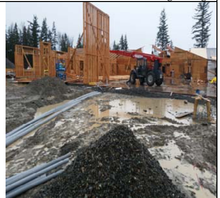
Electrical Connection To Electrical Room
