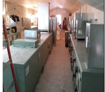
...More Heating/Ventilation Units
