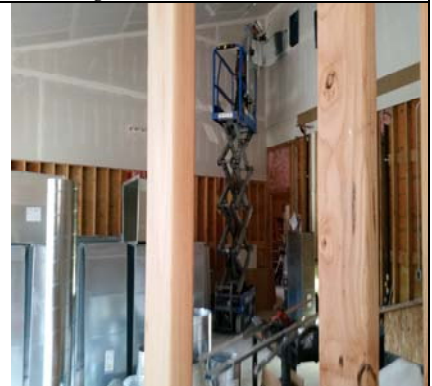
HVAC Ductwork Classroom Connections
