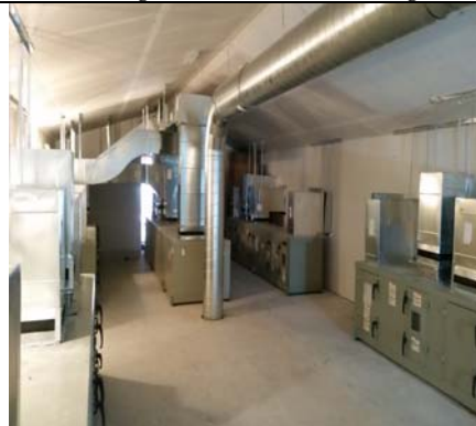
Heating/Ventilation Ductwork In Mezzanine
