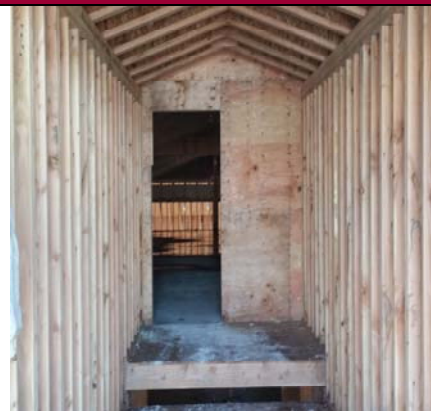
Mechanical Mezzanine Hall Connector
