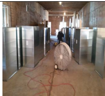
...More Overhead Ductwork Down The Hall
