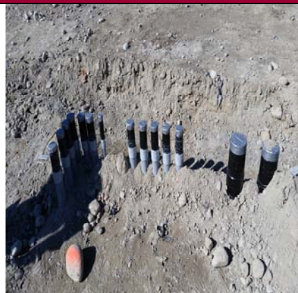
IDF In Ground Computer Line Distribution
