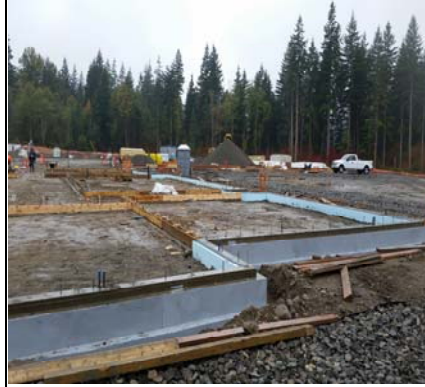
Interior Footings Needing Concrete
