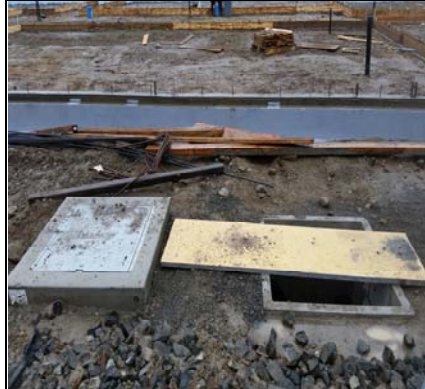
In-Ground Vaults For "Future" Portables
