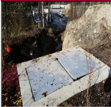
Main Power Vault Up By Swenson Ave
