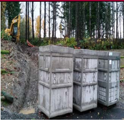
On Site Power Distribution Vaults & Ditch
