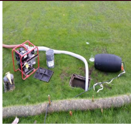
More Pumps & Pipe Management Bladders
