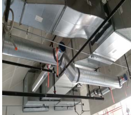
East/South Wings - HVAC Air Intake Ductwork
