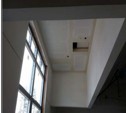
Light Wells - Sprinkler Head Access
