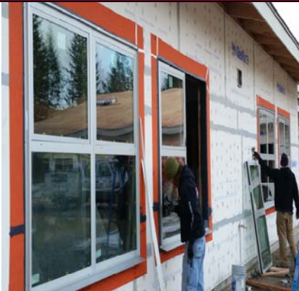
Air/Water Barrier Window Seal - Windows
