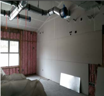
Batt Insulation - Sheetrock - Ductwork
