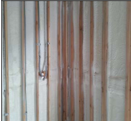
Interior Wall Foam Insulation
