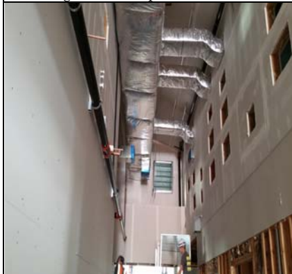
Admin Wing - Library Hallway HVAC
