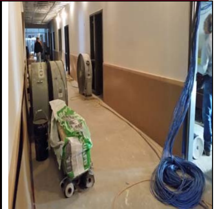
Main Hallway & Telecom Room
