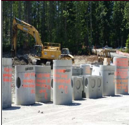
Sanitary Sewer & Drainage Structures
