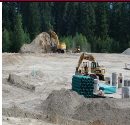
Piping & Drainage Structures
