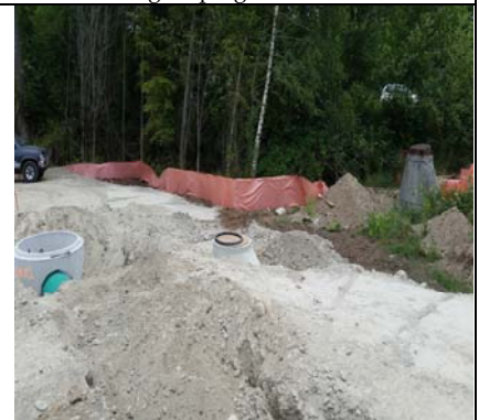
Storm & Sewer Drainage Structures
