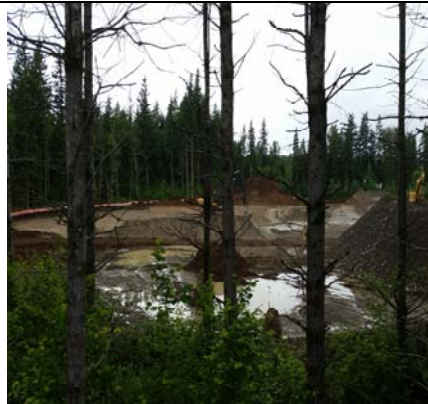
Contained Surface Water 2- 6/2 & 6/3
