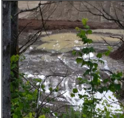
Contained Surface Water - 6/2 & 6/3
