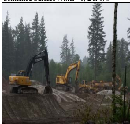
Equipment Shut Down - 6/2
