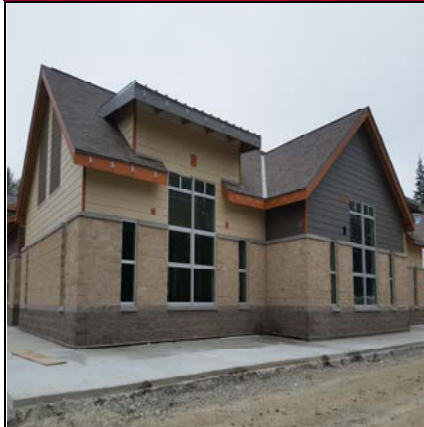
Pending Gutters And Landscaping
