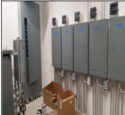
Electrical Sub-Feed Power Distribution
