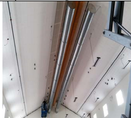
Gym-Acoustical Ceiling-Ductwork-LED Lights
