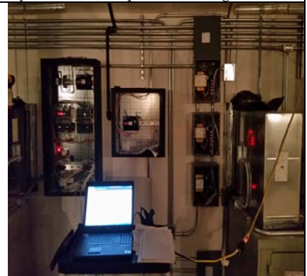
Building Automation Coming Online
