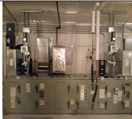
HVAC Bumped - Pending Startup
