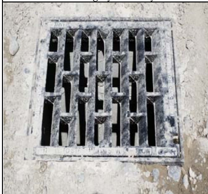
Catch Basin Ready For Silt Protection
