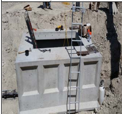
Main Water Vault 2
