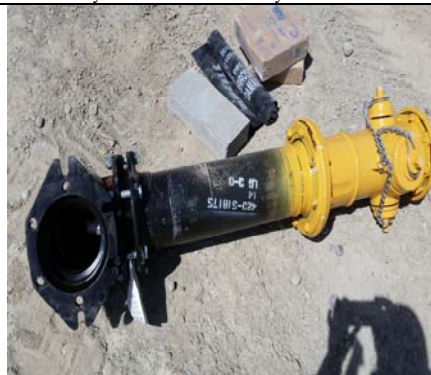
For The Fire Hydrants
