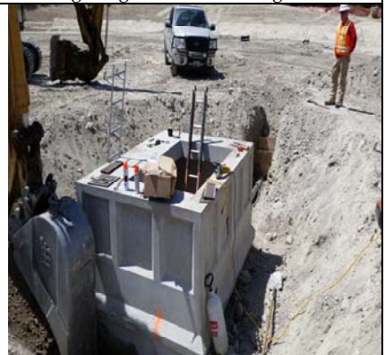
Main Water Vault
