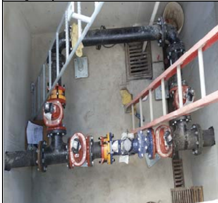
Water Main Vault & Valves
