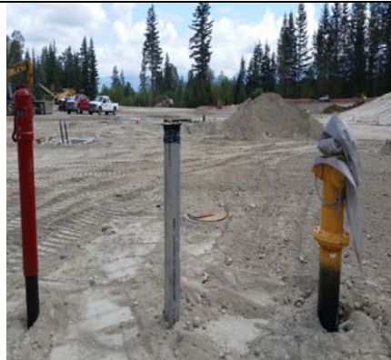
Post Indicator/Fire Department Connection
