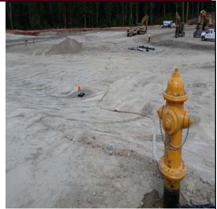
Fire Loop Fire Hose Flush To Pond
