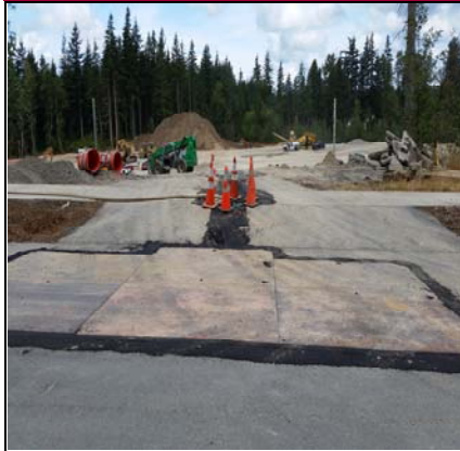
Fire Loop Connection Point
