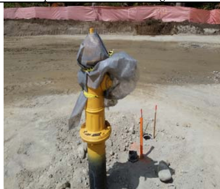
Fire Hydrant Protection
