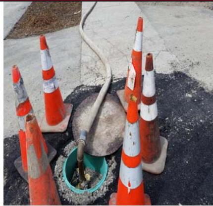
Fire Loop Flush Point For Testing
