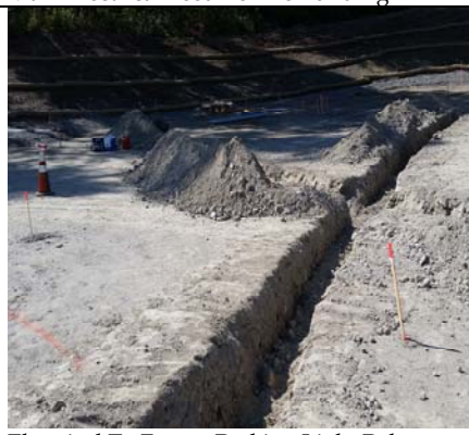
Electrical To Future Parking Light Pole
