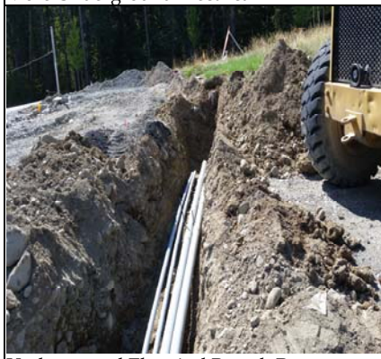
Underground Electrical Branch Runs
