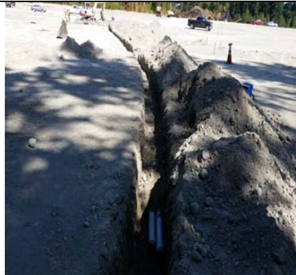
Main Electrical Feed To The Building
