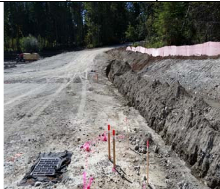
Underground Electrical At Bus Entry
