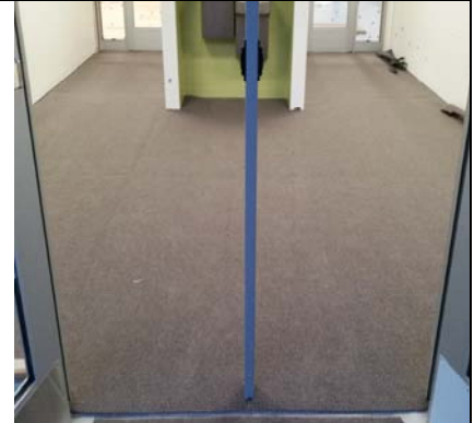
"Walk-Off" Carpeting Installed At Entries
