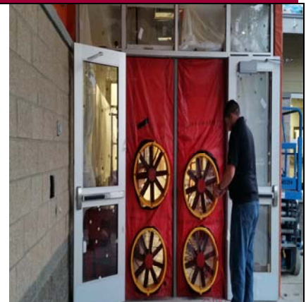
Fans Setup In Main Entry And NW Wing
