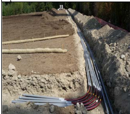
Underground Electric & Telecom 2
