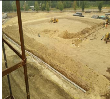
Underground Power - North Parking Lot
