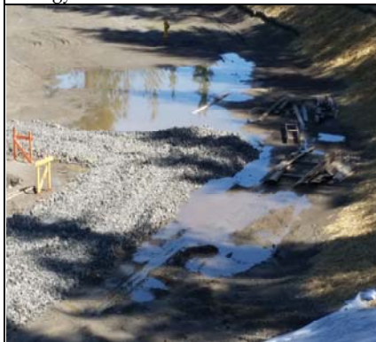
Holding Water On Site After The Rain
