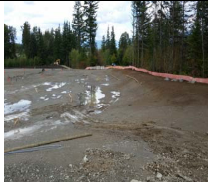
Because Of Holding Surface Water On-Site
